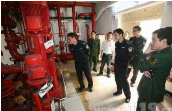
Firefighting facility issues
